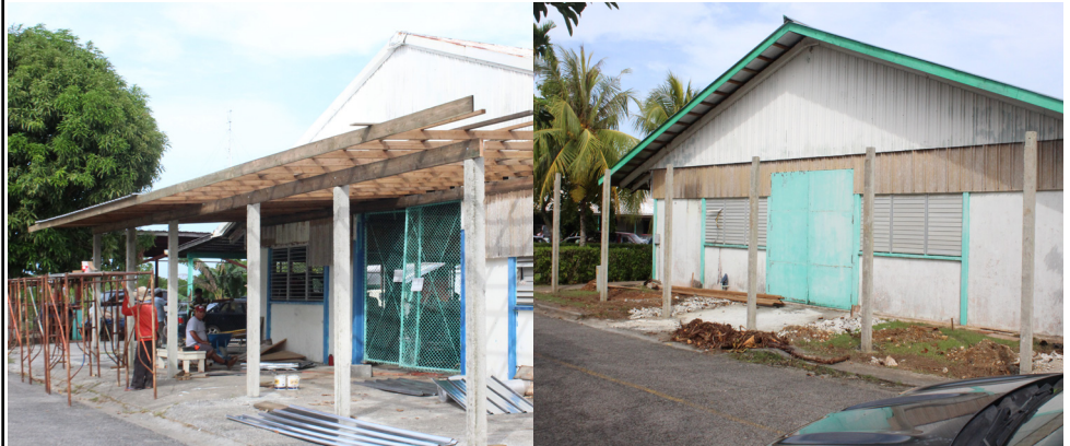
Automotive Mechanic Technology and General Electronics Technology Shops small scale project near completion.
