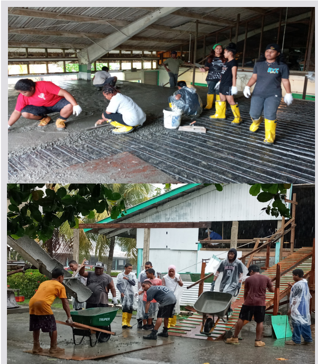
PCC CTE Lab School students cementing the 2nd floor of Tekrar Building for additional PCC classrooms on Tuesday, April 28, 2020.
