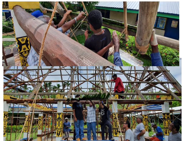
CTE students get a first hand experience in roofing Mesekiu Bai from their instructor President Dr. Tellei
