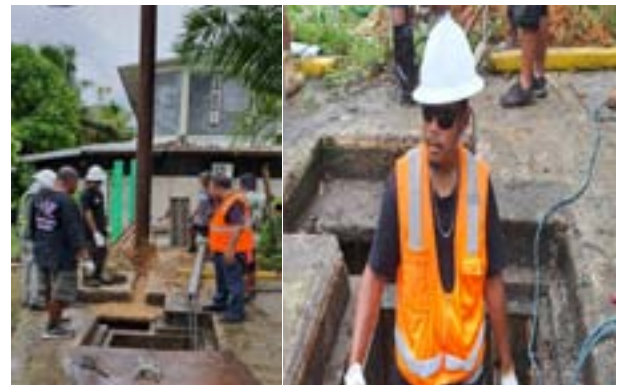
left: PPUC crew connecting conduit pipe to the new powerline pole. right: Blake Yuri a former PCC GE students connecting underground power line. PCC thanked PPUC and Maintenance for working diligently to ensure PCC's Administration bldg electrical power get back online.
