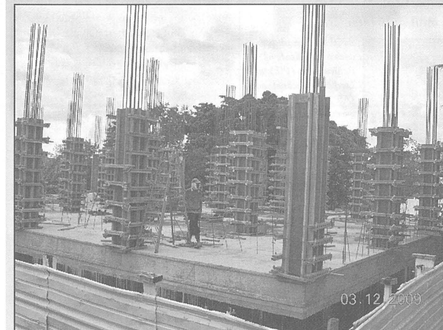
Construction work is progressing on schedule with the second floor columns already going up.
