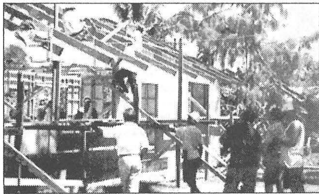
PCC construction students and crew putting up the roof of Palau High School's new Math Building.
