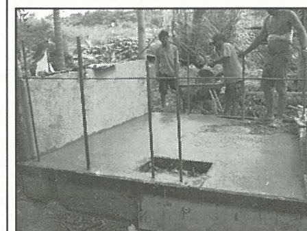
Construction of the Dry Litter System pilot project at John Oiph's farm in Ngerikiil, Airai.
