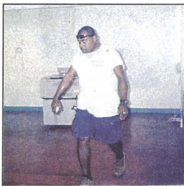
Crew Leader Willes Tmecherur inspects work on the new classroom that previously served as the Adult High School Office
