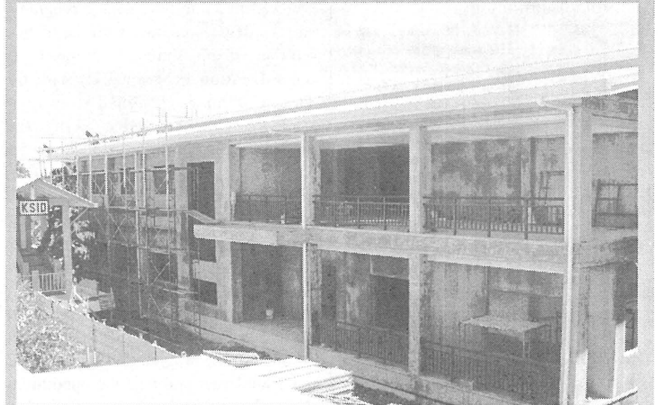
With 93 days left on the construction schedule, work on the interior walls and ceilings is finished. Workers are now preparing the outer wall for painting. The newly constructed three-story building will house the library collections on the first two floors while the top floor will be used for faculty offices and the ASPCC office.
