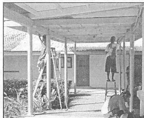
Maintenance workers painting the trimmings, giving a new look to the campus.
