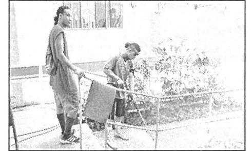
Albino Esoailug assisting Charles Tachibemmel pull the hose as the water blasting continues down the stairs.
