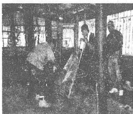
Vincent Bayow and George Fagalen pouring cement for the new chicken house floor and their Masonry Instructor, Besechel Kiuluul.
