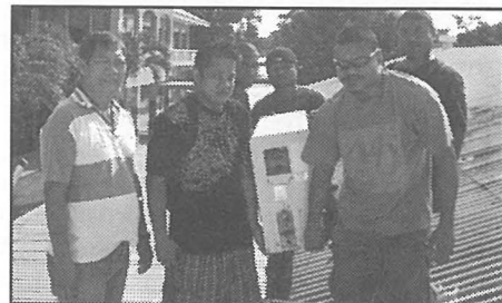
The morning AC class removing the final air conditioning unit from the roof.
