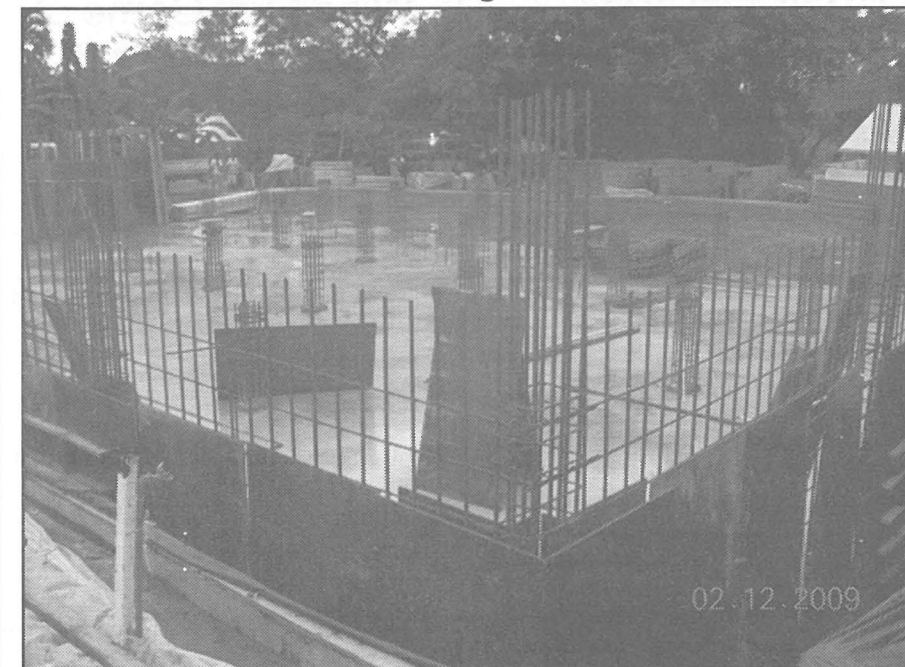
Forty-four (44) days into 270 days of construction, the entire first floor has been poured and work is progressing the first floor retaining wall. Upon completion, the three-story library complex will rival the Btaches Classroom Complex in height, and command a presidential view of the track & field and the surrounding waterfront.
