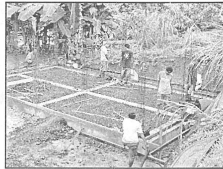
Construction Technology Students and their instructor Lester Rekemesik work on the foundation of a PCC bungalow.
