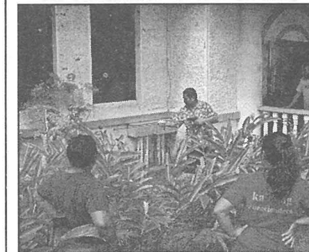
A good crowd gathers around Vice President Olegeriil as he water blasts the outside walls of the administration building during last Friday's general cleanup.
